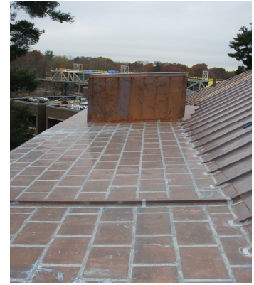
Flat seam copper roof comprised of pans no larger than 18"x24". Note also the expansion batten.
